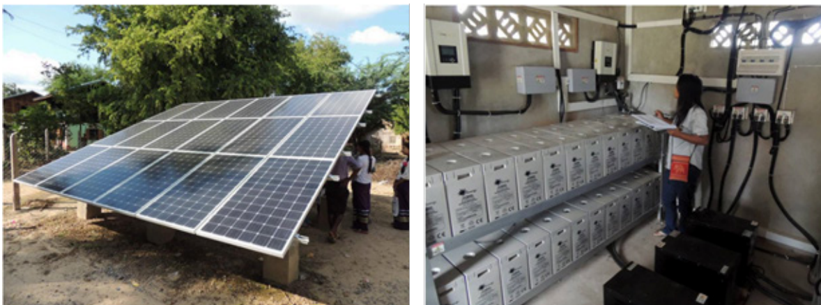
FIGURE 25. Left: a PV mini-grid installed as part of ADB's demonstration of solar mini-grids. Right: battery powerhouse, part of a pilot solar mini-grid.
