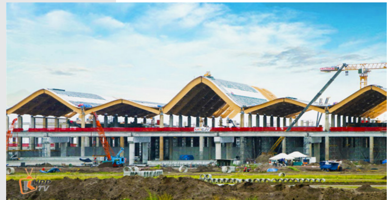
Ongoing construction of Clark International Airport's Terminal 2 (Phase 1) that is expected to start operating in 2020 to accommodate 8 million travellers. Second runway is also in the pipeline (2nd Phase) to accommodate 22 million travellers. Klipp.tv
