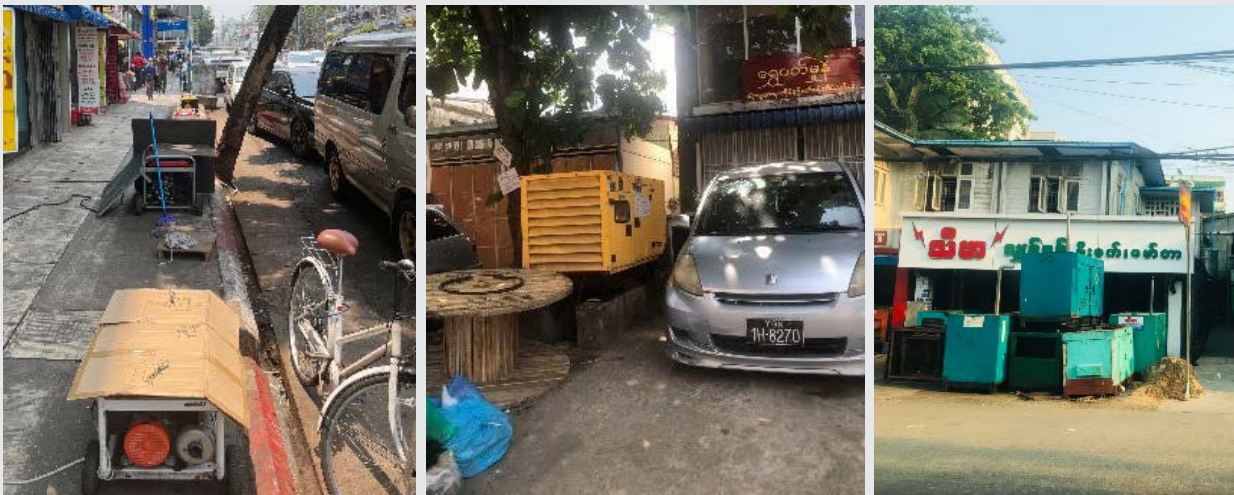
FIGURE 13: Generator alternative power source (Yangon)
