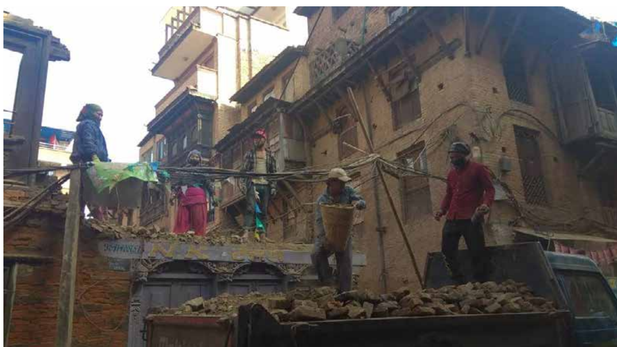
Demolishing and transporting debris in a densely built-up area near Durbar Square in Bhaktapur, November 2019. Photo: Kiran Bhattarai
