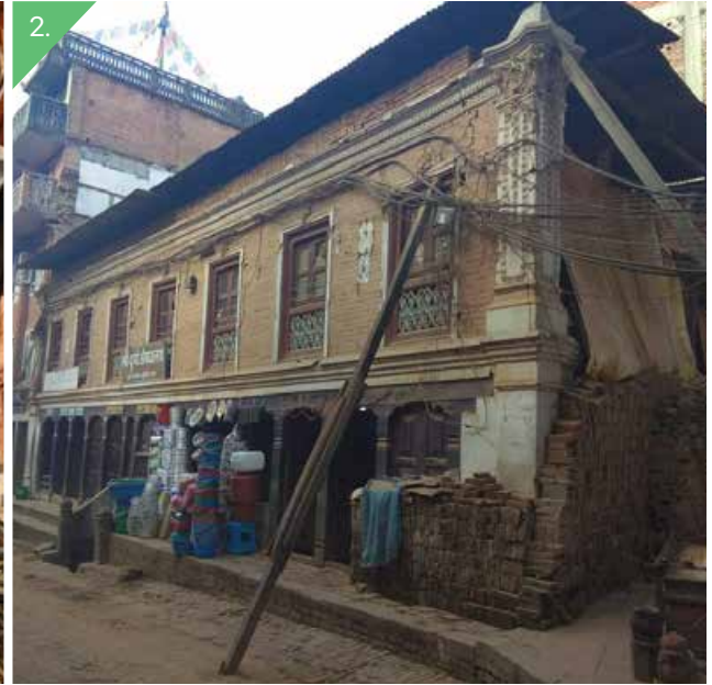
2. Aurvedic medicine shop in earthquake-damaged house in Bhaktapur, November 2019. Photo: Pallavi Payal
