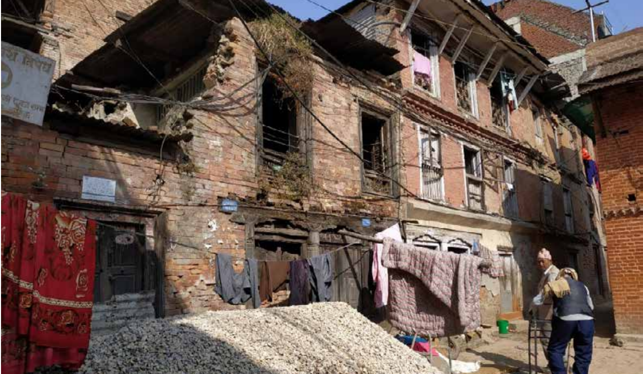
Earthquake-damaged houses in Bhaktapur Municipality, November 2019. Photo: Lena Michaels
