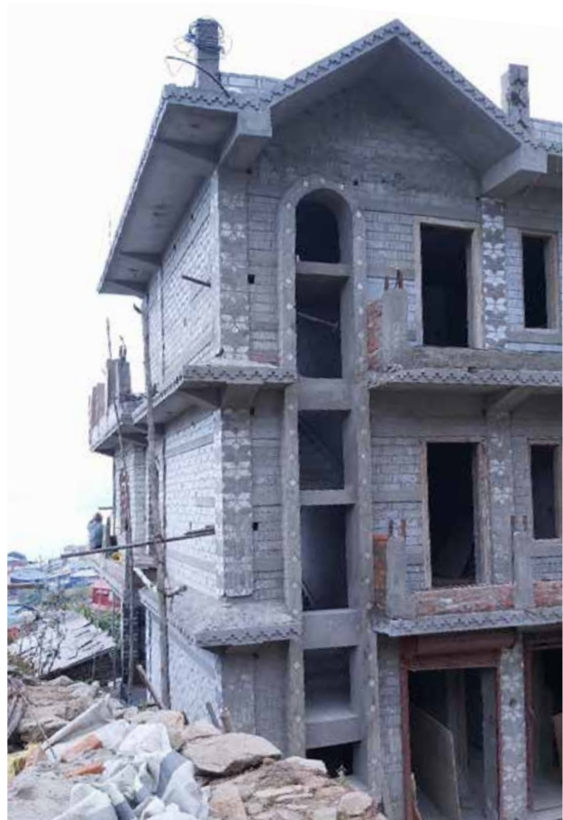
House under construction in Barpak, Sulikot Rural Municipality, Gorkha, November 2019. Photo: Manasi Prasai
