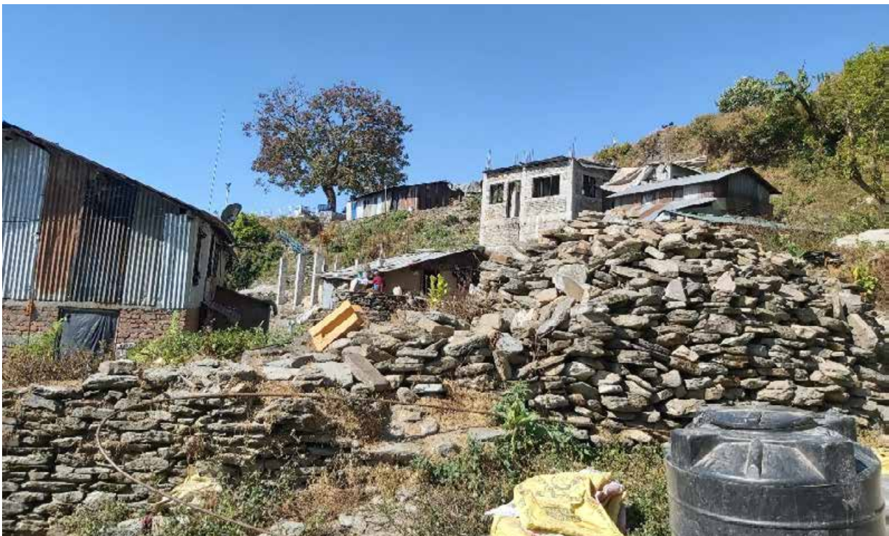
Remnant of earthquake damage and new houses under construction in Gairhigaun, Barpak, Gorkha, November 2019. Photo: Manasi Prasai
