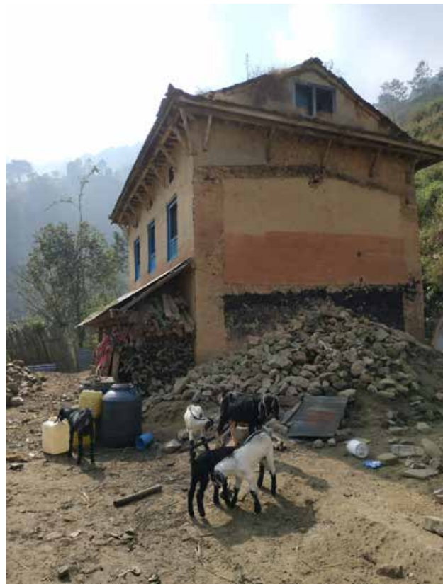
Damaged house in Suryabinayak, Bhaktapur, 2019. Photo by Lena Michaels
