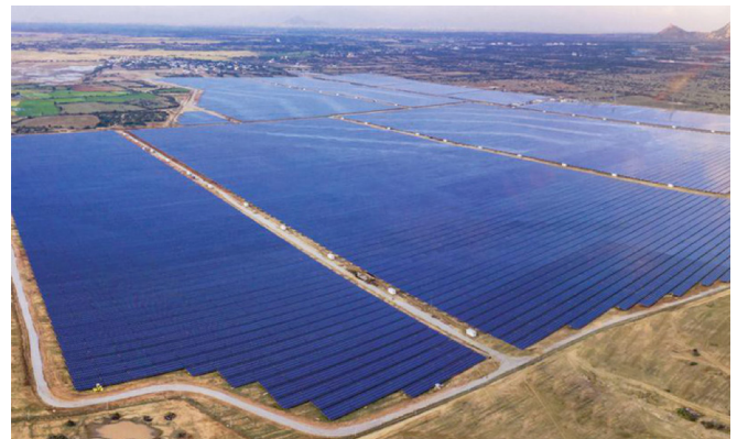
Photo 1. A large solar facility in Ninh Thuan Province.
